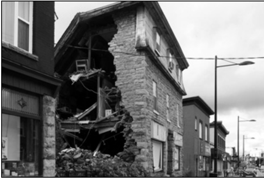
Magee House partial wall collapse and emergency demolition
