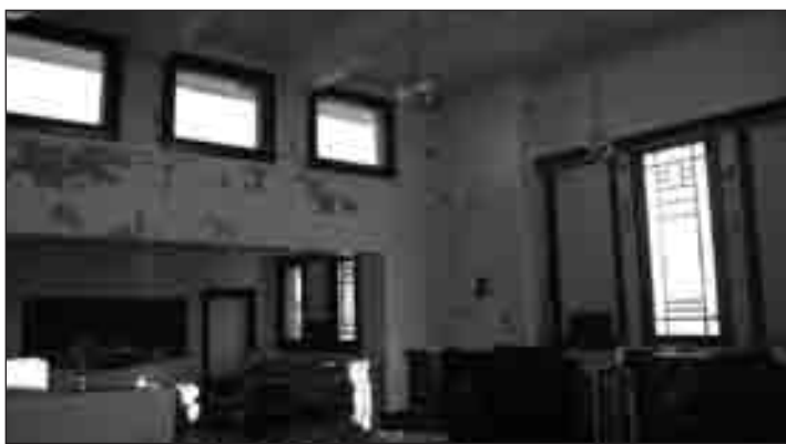
Interior of the upper front level of the building, what would be called the banquet hall. Original prairie style designs embellish some of the windows.
