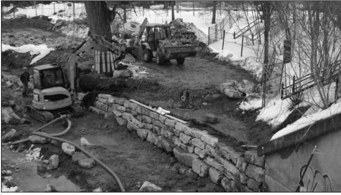
North side of Patterson's Creek Pond showing first portion of stone retaining wall being reassembled.
