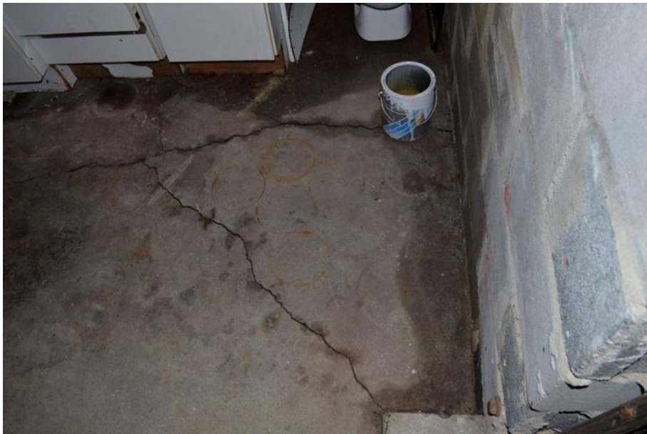
Cracks in floor slab
