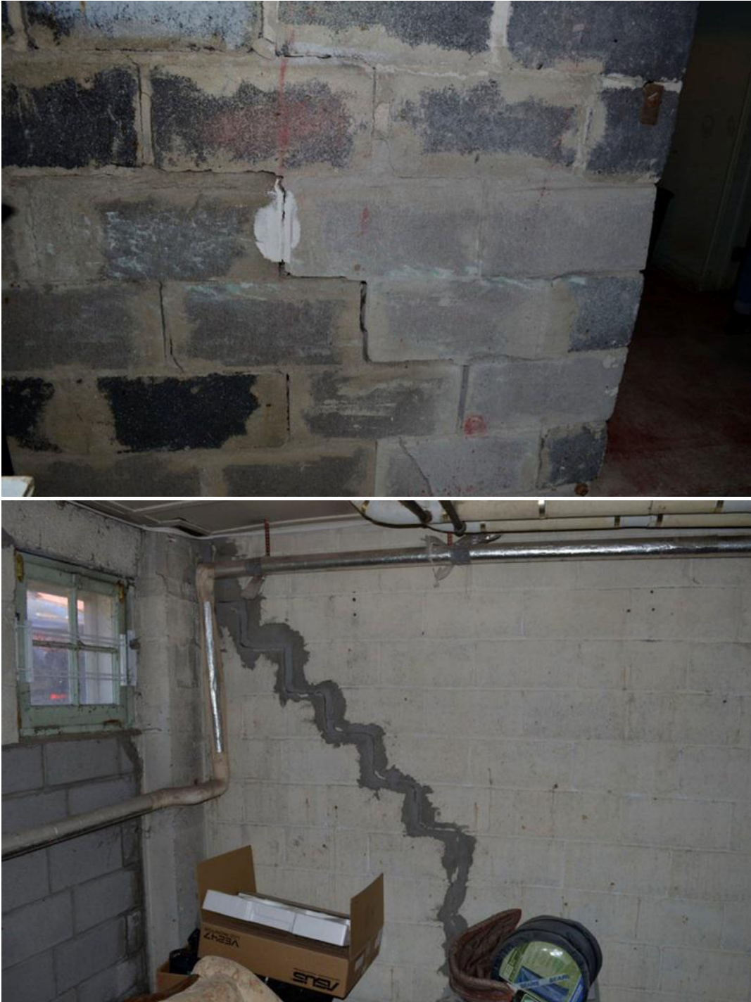
Cracking in foundation wall
